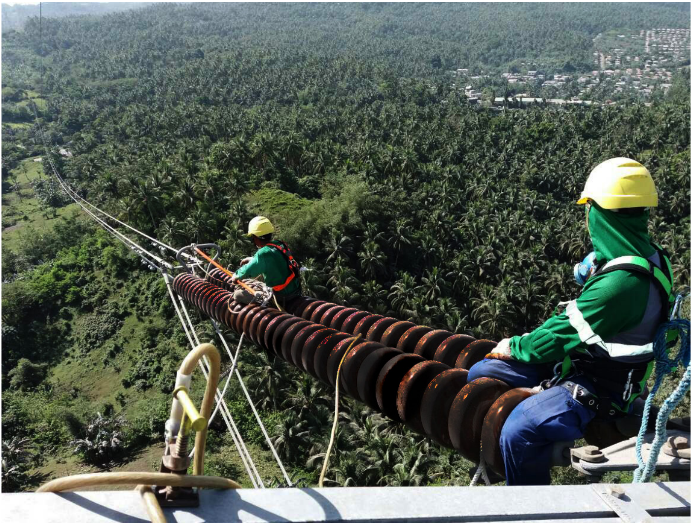
Besides the submarine cable connecting Mindanao to Visayas, over 185 kilometers of overhead power lines will also be used to connect transmission facilities in the area.
