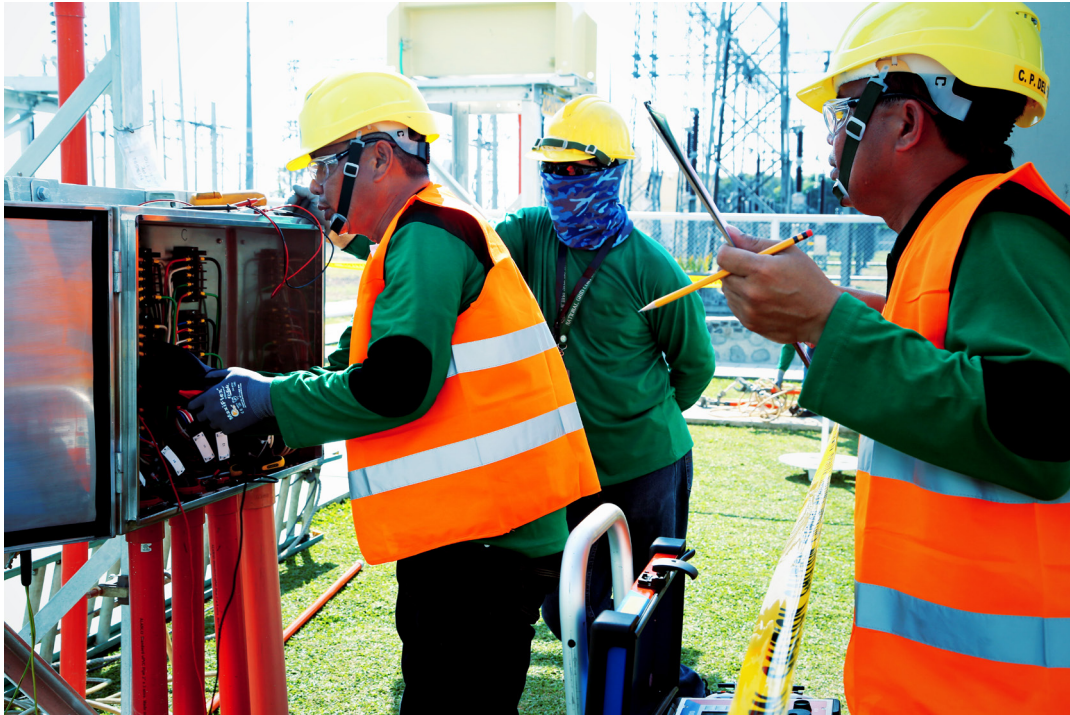
Personnel from the Maintenance and Testing Division (MTD) ensure the reliability of the grid's equipment and facilities to maintain the smooth transmission of power.
