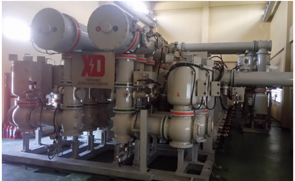
NGCP's new 230-kiloVolt Gas Insulated Switchgear (GIS) in its Las Piñas Substation will supply the power requirements of Las Piñas, Cavite, Parañaque, Malibay, Pamplona, Imus, Bacoor, and Metro Manila areas. The new GIS, along with a new 300MVA transformer, was energized on May 28 and June 5, 2017, respectively.
